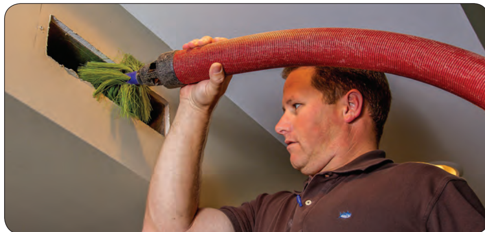
Ducts may need to be serviced by professionals in homes where indoor air quality is poor.
