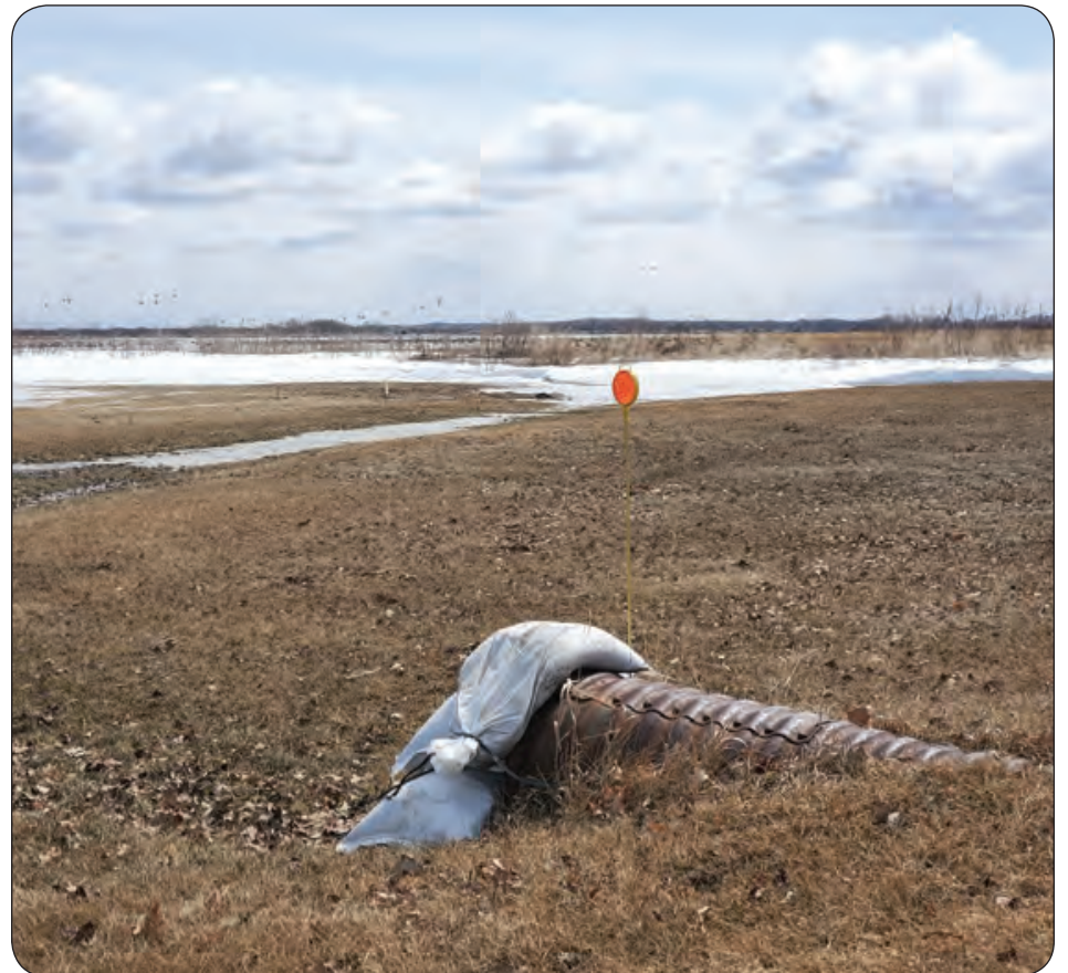
The RM of St. Andrews Public Works block off a culvert at a home on Minchull Road in Clandeboye on April 12.
