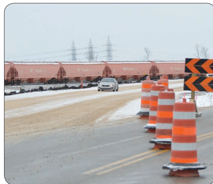
RECORD PHOTO BY DAVE BAXTER A car makes its way down a new gravel section along Highway 204 last Thursday afternoon. A 600 metre section of the St. Clements Highway, just south of CIL Road, otherwise known as Highway 509, has been shifted 60 metres to the east of the Red River. The $1.3 million project, which is being fully funded by the provincial government, will be completed once the road is paved sometime next summer.
