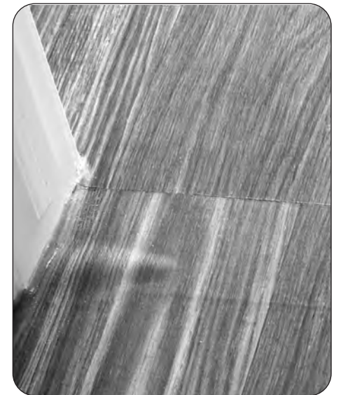
Bubbling flooring and lack of transition to a bedroom.
