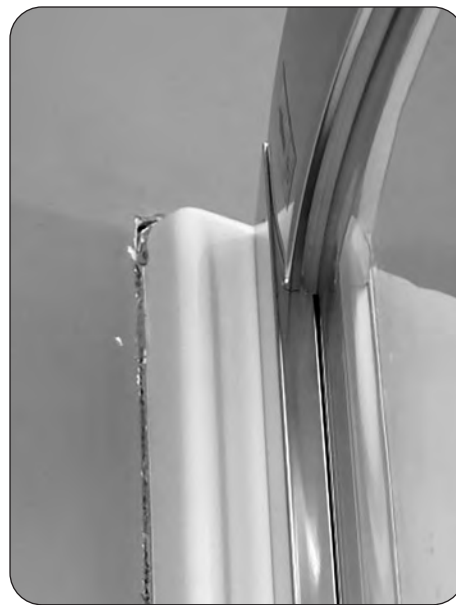
The shower was left unsealed.
