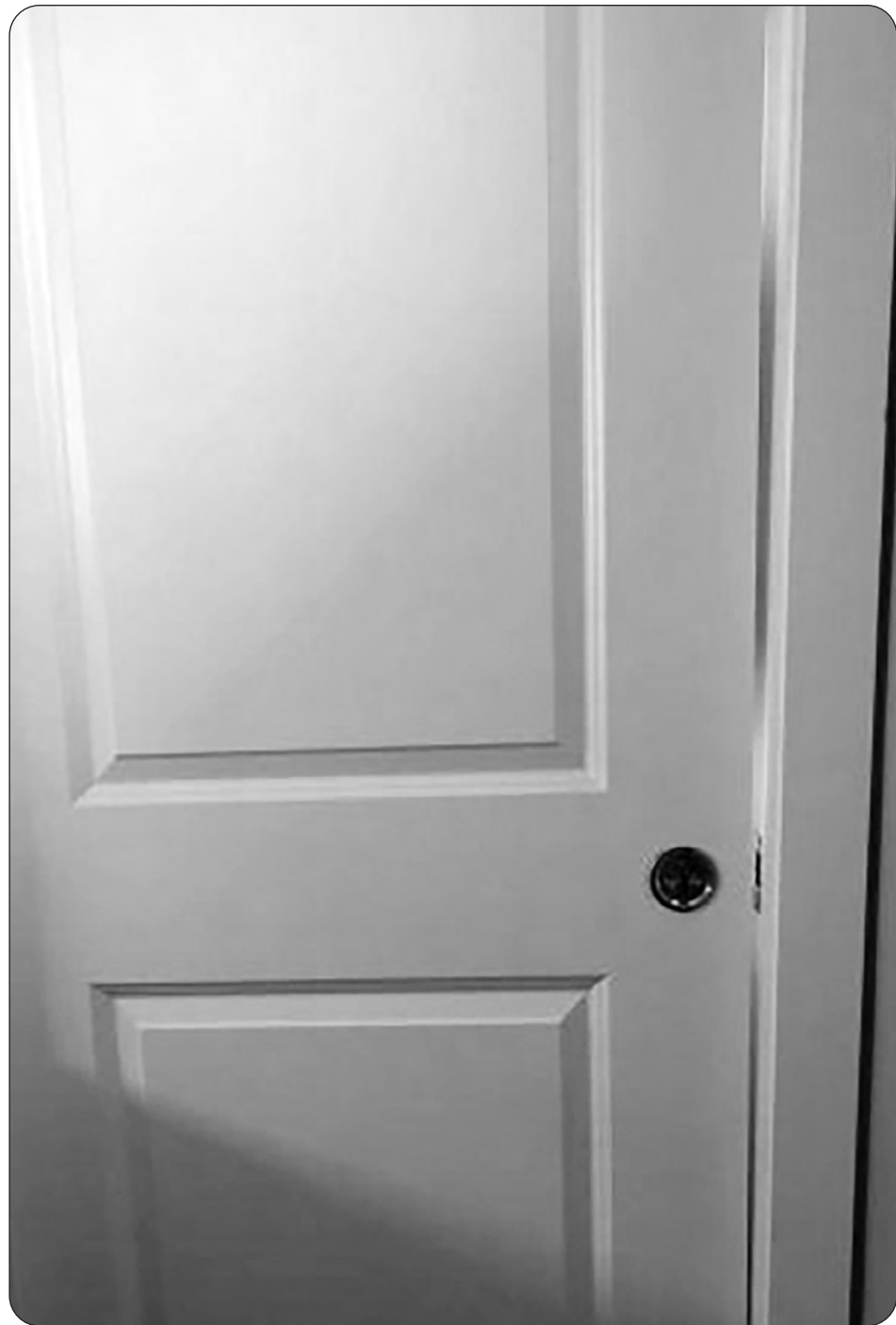
One of the doors that wouldn't close properly.
