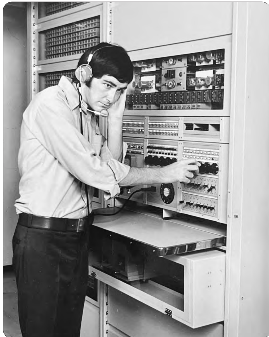
An employee of AEI Telecommunications with the racks, that contain the switching equipment for the earlier versions of the control boards.
